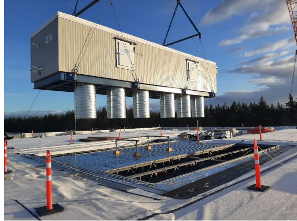
An A+P Insulated Penthouse Evaporator being installed on the roof of a refrigerated grocery distribution center. Similar industrial exterior components were used for the refrigerated trailer manufactured for the N.E.W. Cool Pup Trailer.
