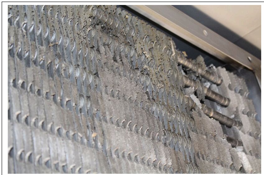
Figure 7: Aluminum fins severely corroded by application of highly alkaline (pH > 9.0) cleaning chemicals.
